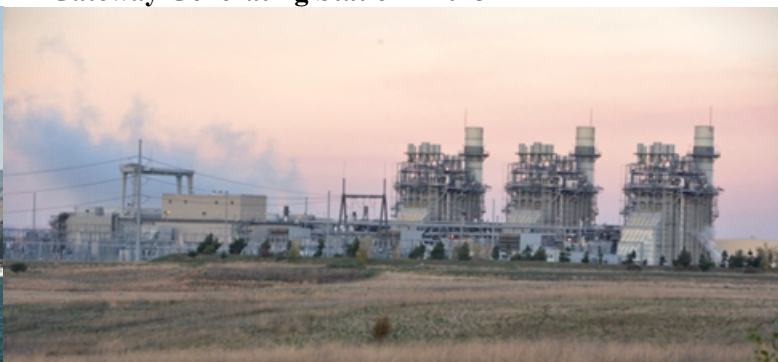
Delta Energy Center - 2016
