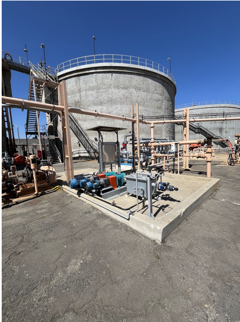
Interim FOG Receiving Station
