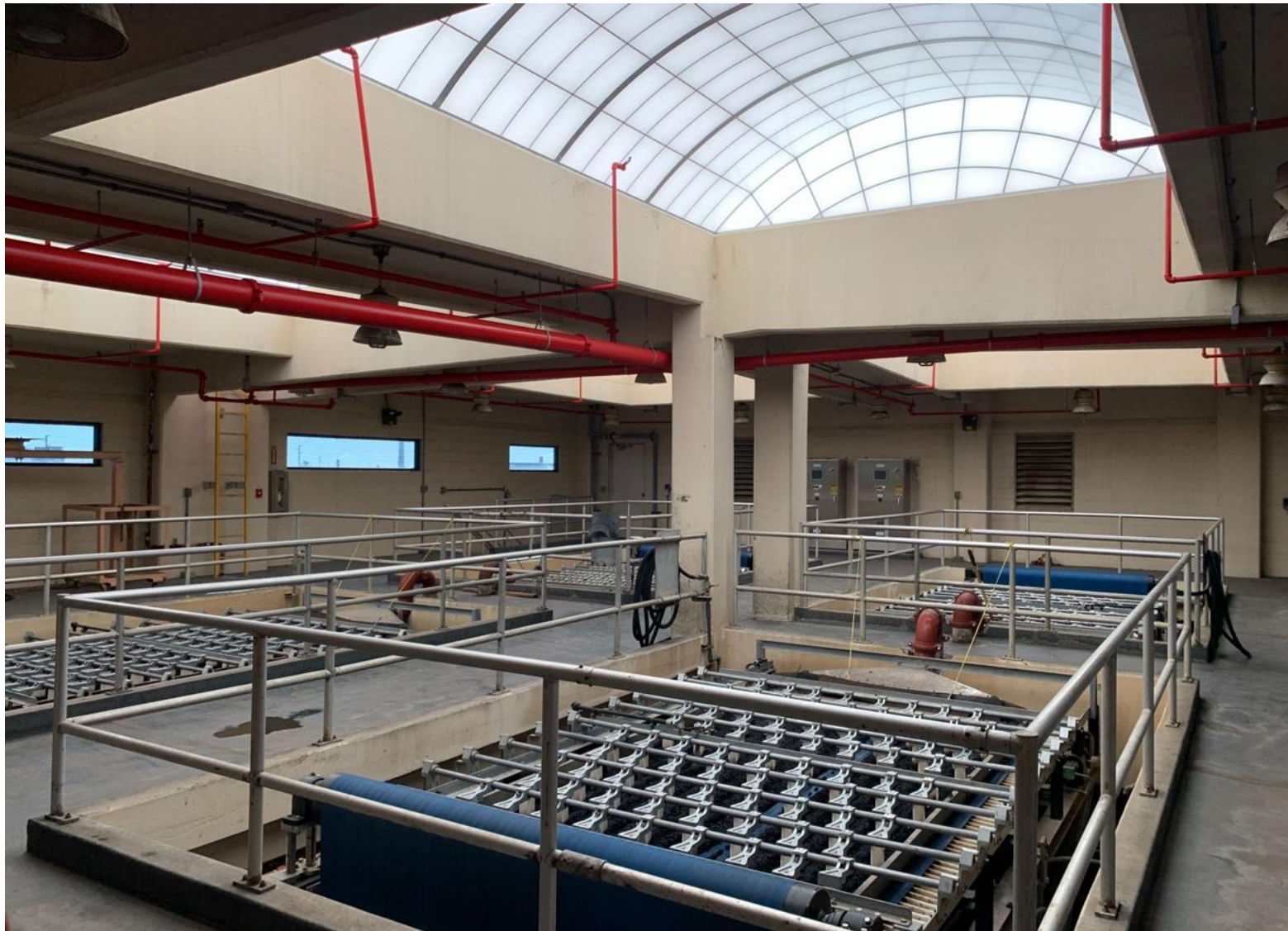
Dewatering of sludge using belt filter presses
