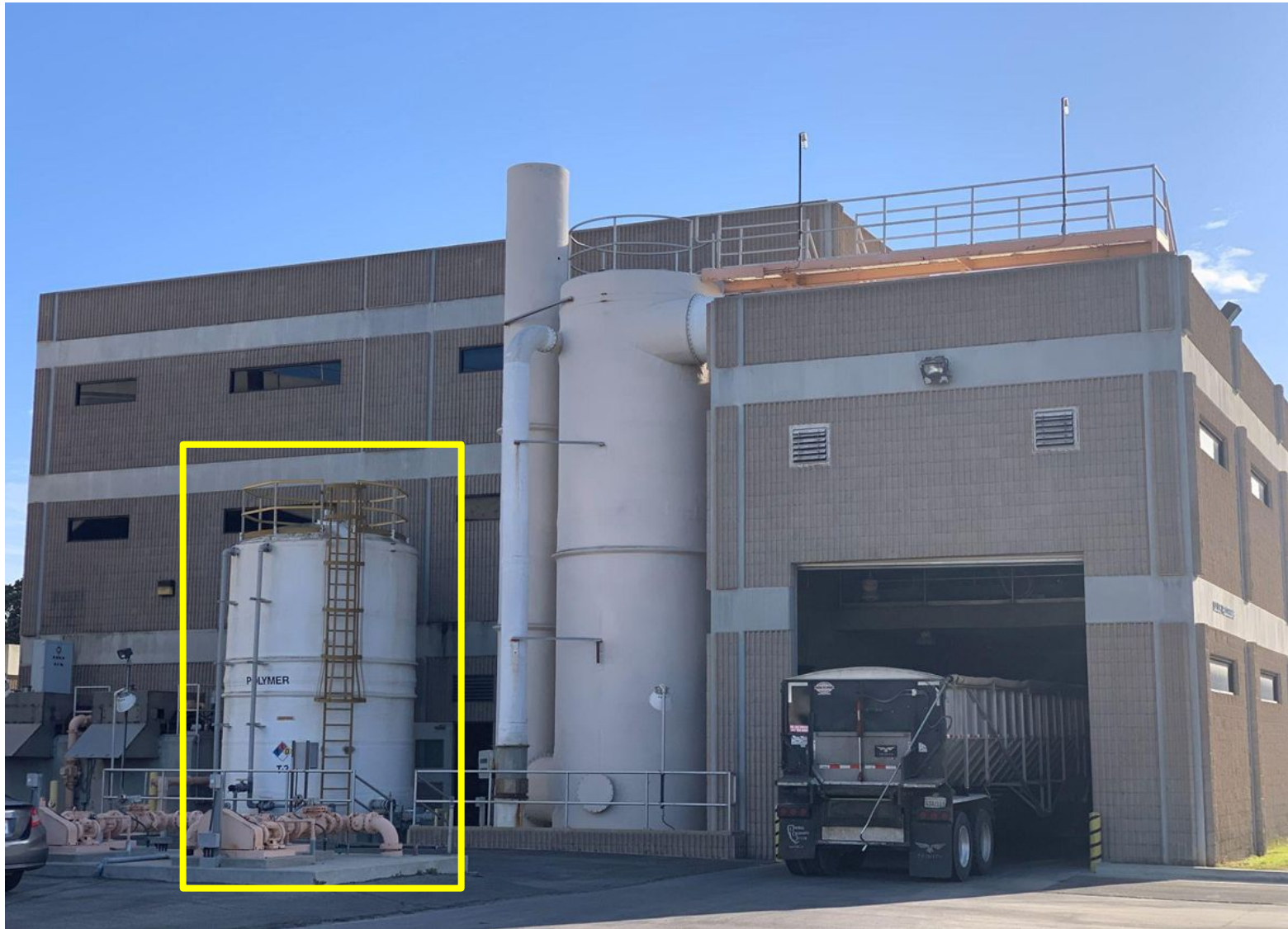
Polymer storage at the Wastewater Solids Processing Building 252
