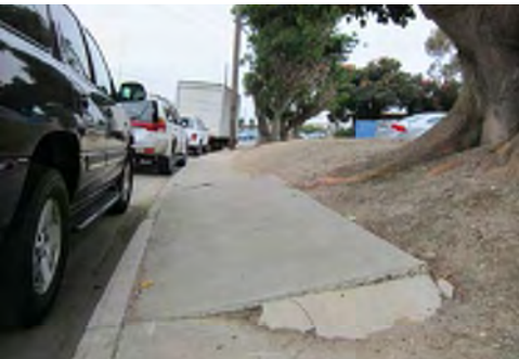
Tree roots damage a sidewalk on Richmond Avenue.
