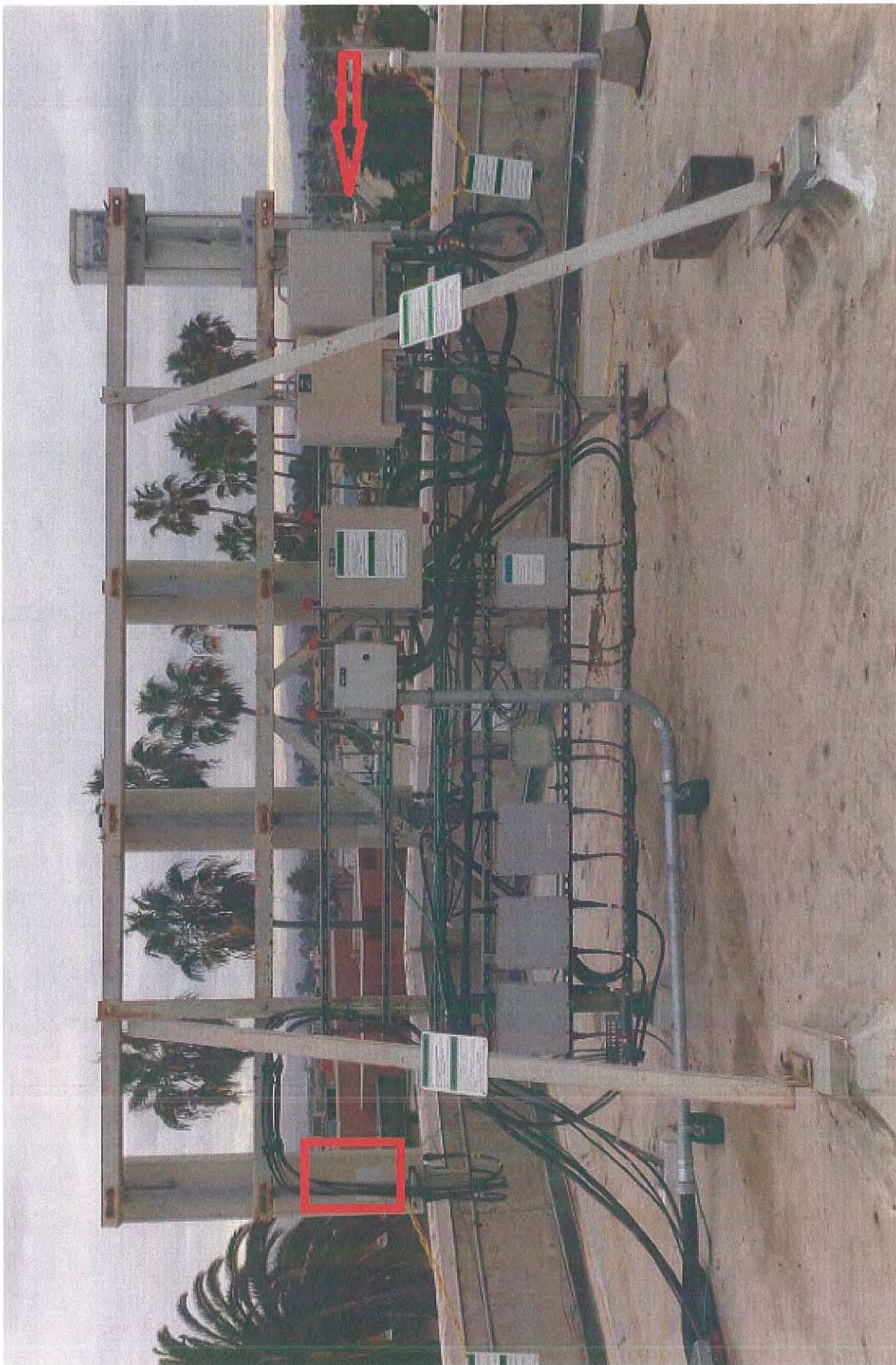
Attachment #3: Photograph of Existing Equipment Rack
