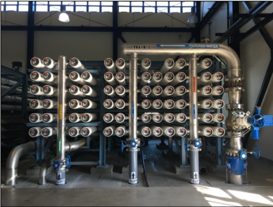
Reverse Osmosis Train
