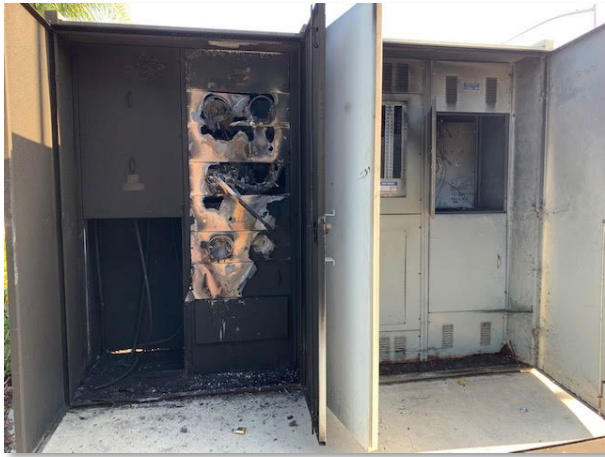
Damage from September 2019 fire
