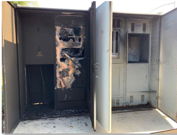
Damage from September 2019 fire
