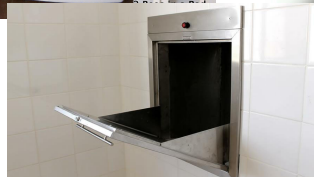
TRASH CHUTES AT EVERY FLOOR LEVEL
