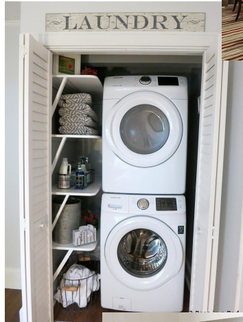
WASHER DRYER UNITS AT EA UNIT
