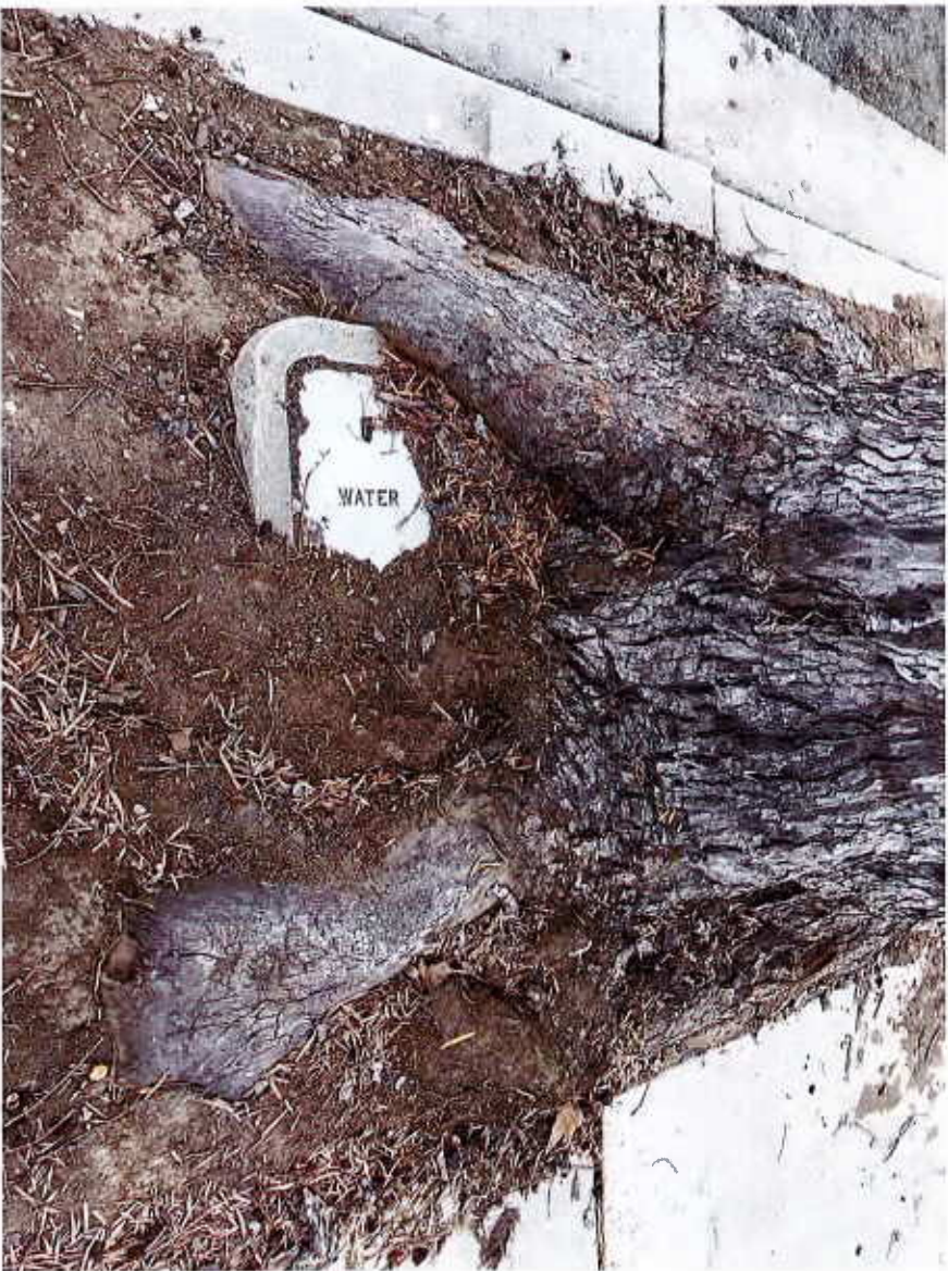
Exhibit 2. Tree root conflict with a water meter box as a result of improper spacing.
