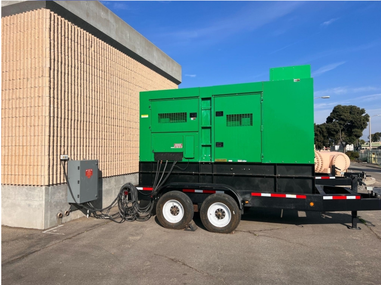
Backup Generator Switch (Interstage Pump Generator)
