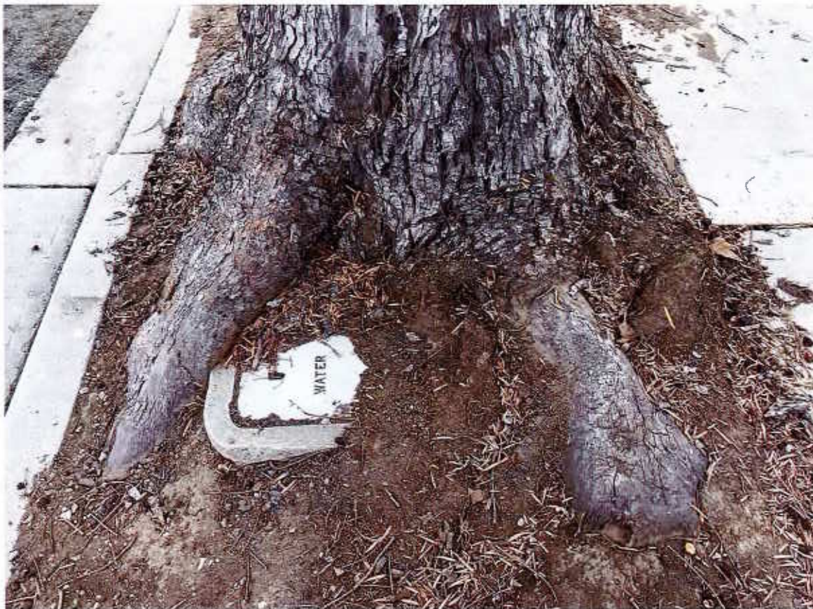
Exhibit 2. Tree root conflict with a water meter box as a result of improper spacing.
