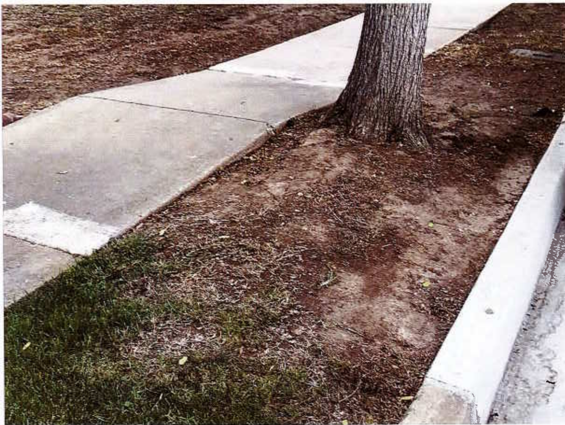
Exhibit 1. Tipu ( Tipuana tipu ) planted in a 4.5-foot parkway displacing a sidewalk.
