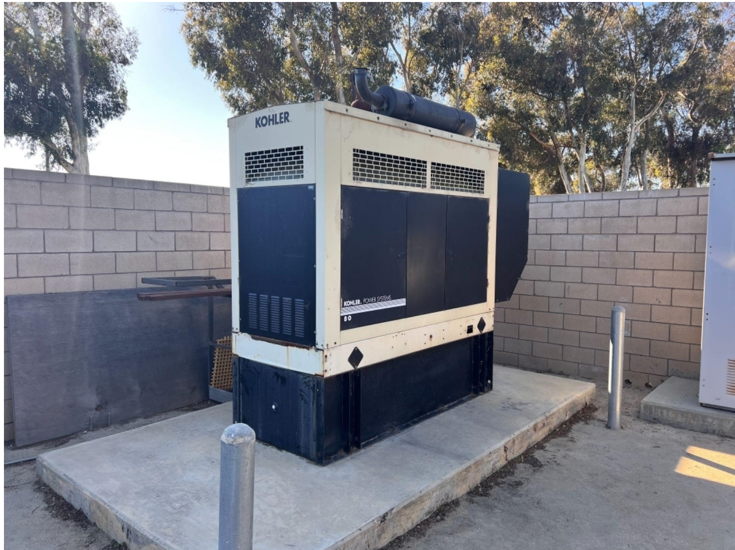
Diesel generator for lift station 28
