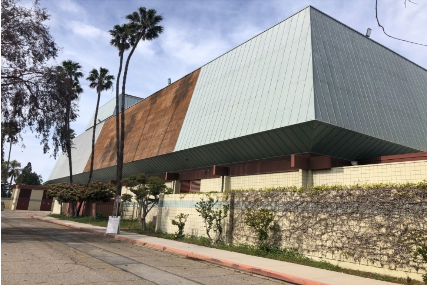
Windstorm damage to Oxnard PACC theater roof.
