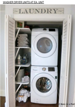
WASHER DRYER UNITS AT EA UNIT
