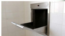
TRASH CHUTES AT EVERY FLOOR LEVEL
