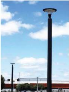
SOLAR WALKWAY LIGHTING
