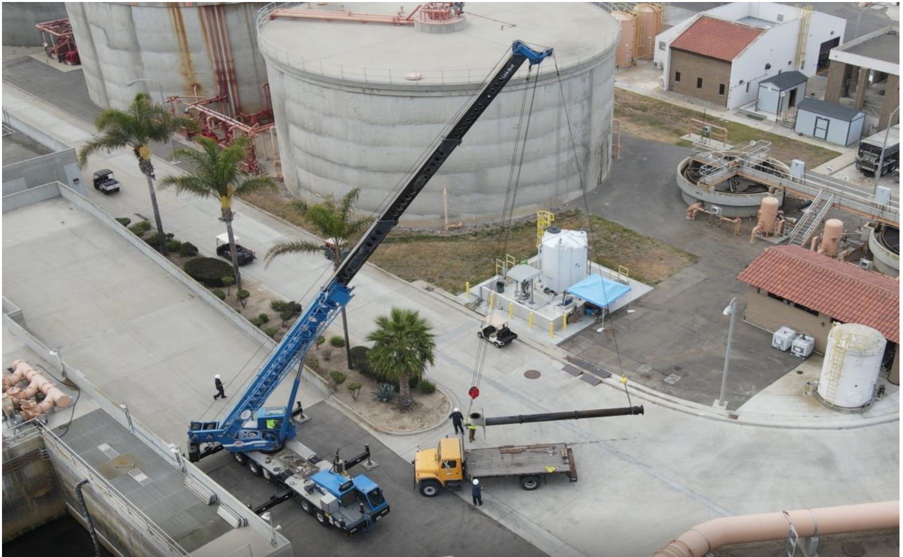
Loading of pump for service request
