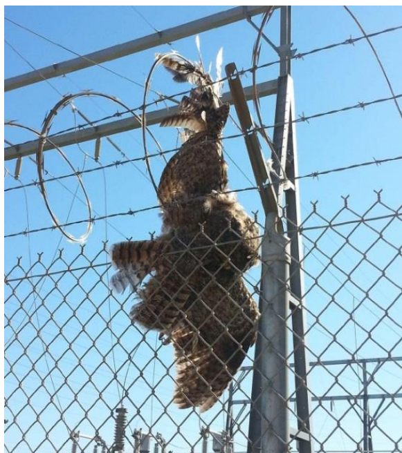
Photo 23. A great-horned owl died after becoming entangled on the razor wire placed on top of this cyclone fence surrounding a substation in Alameda County. Photo by Joanne Mount.
