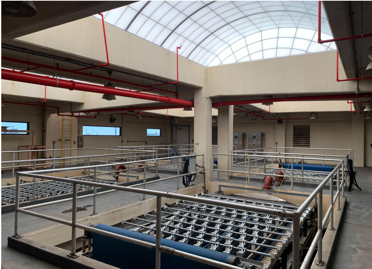
Dewatering of sludge using belt filter presses
