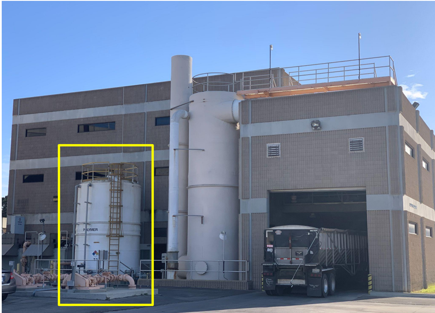
Polymer Storage at Solids Processing Building
