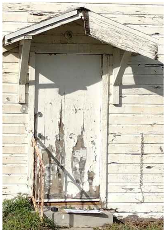
EXISTING ENTRY DOOR: TO BE REMOVED & REPLACED
