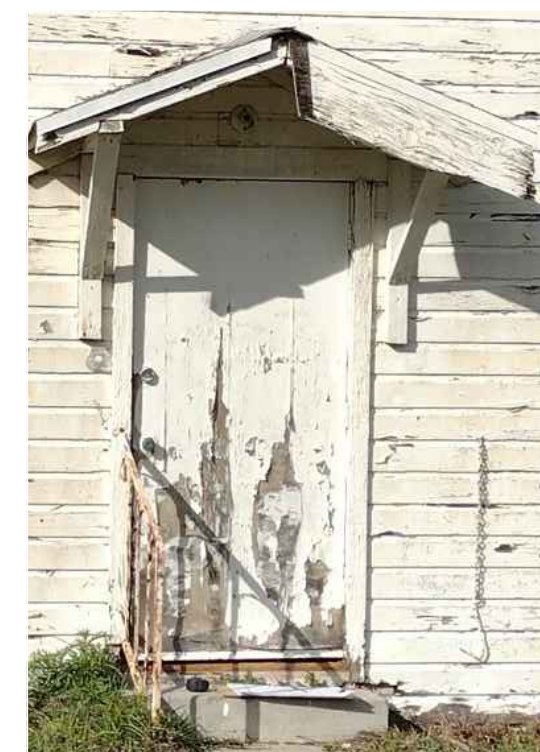
EXISTING ENTRY DOOR: TO BE REMOVED & REPLACED
