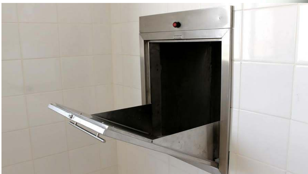
TRASH CHUTES AT EVERY FLOOR LEVEL
