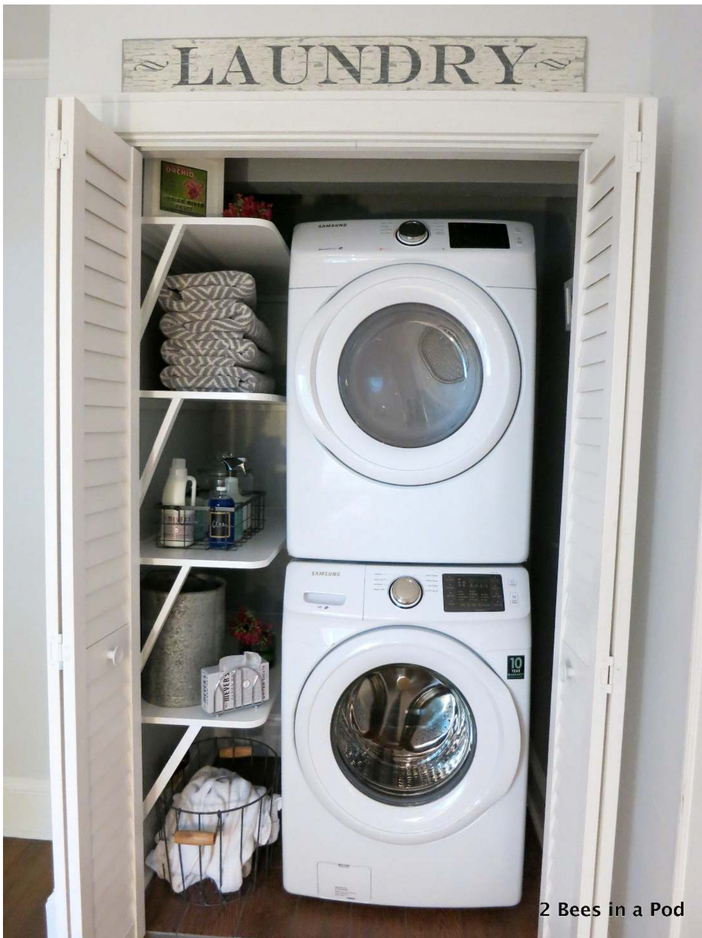
WASHER DRYER UNITS AT EA. UNIT
