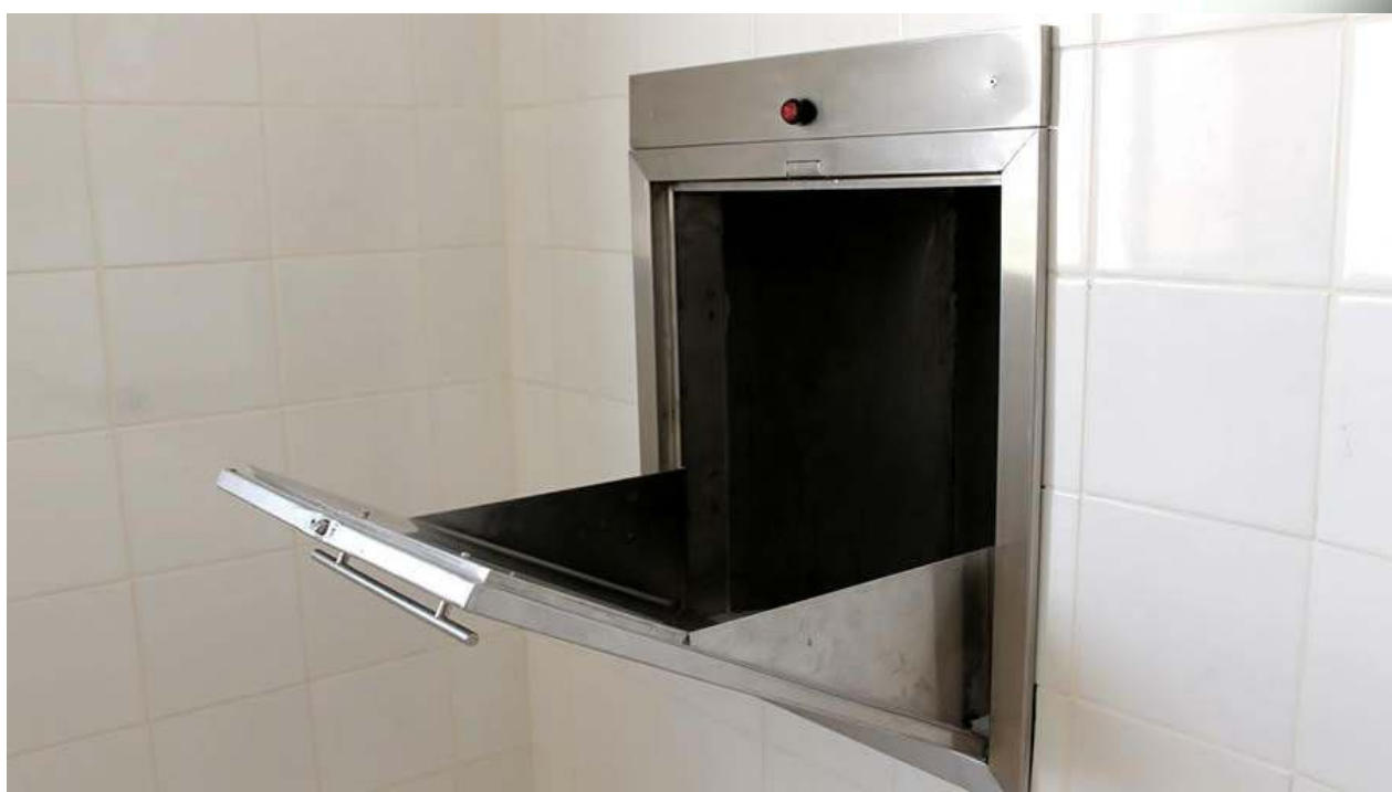
TRASH CHUTES AT EVERY FLOOR LEVEL
