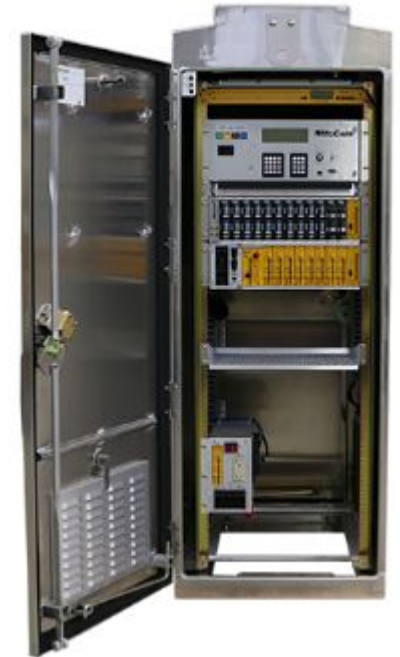
Traffic Signal Cabinet
